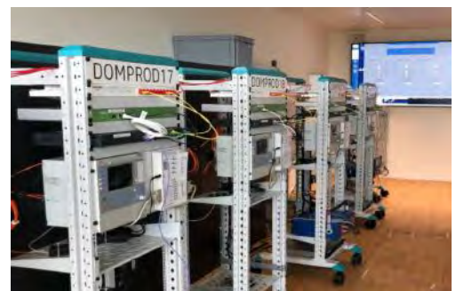
Krinflab: Reconstruction of a Swiss energy substation for the development of attack and defence strategies.
